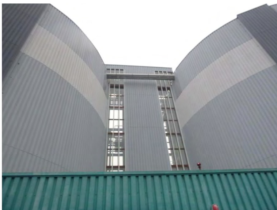
Foto F70, Coating - Slippistingstank 1 & 2
