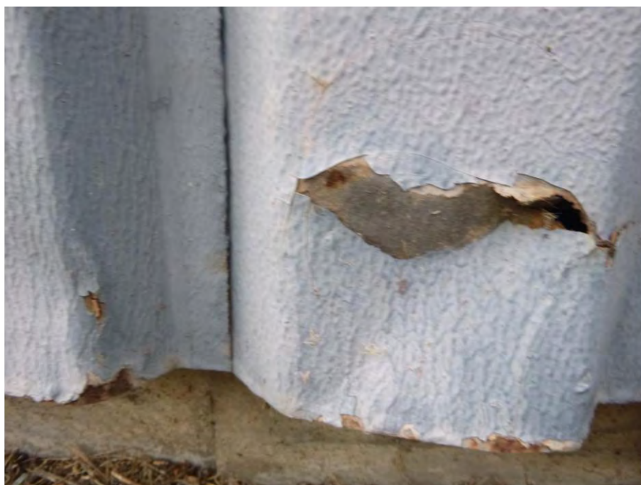
Foto F68, Coating - Slippistingstank 1 & 2
