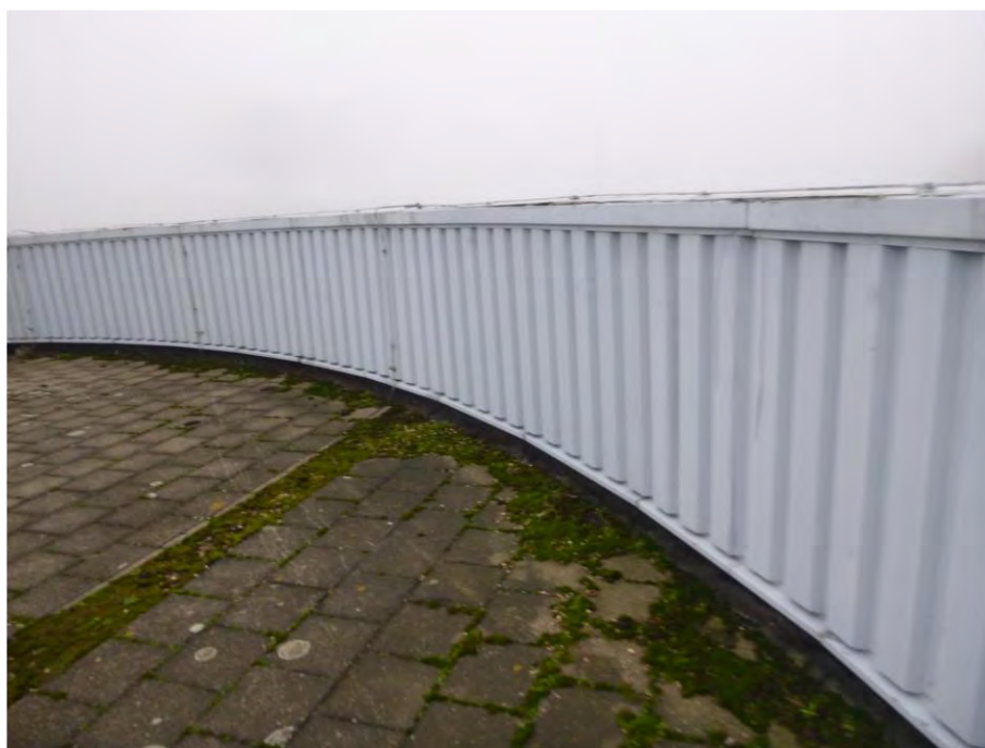
Foto F74, Coating - Slippistingstank 1 & 2
