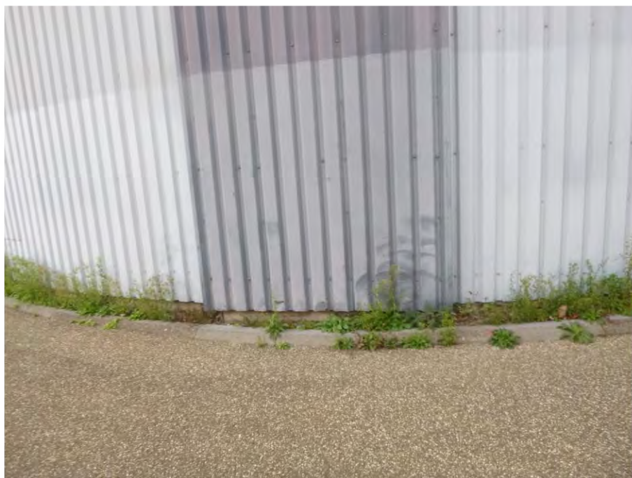
Foto F69, Coating - Slippistingstank 1 & 2
