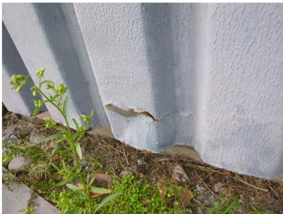
Foto F67, Coating - Slippistingstank 1 & 2
