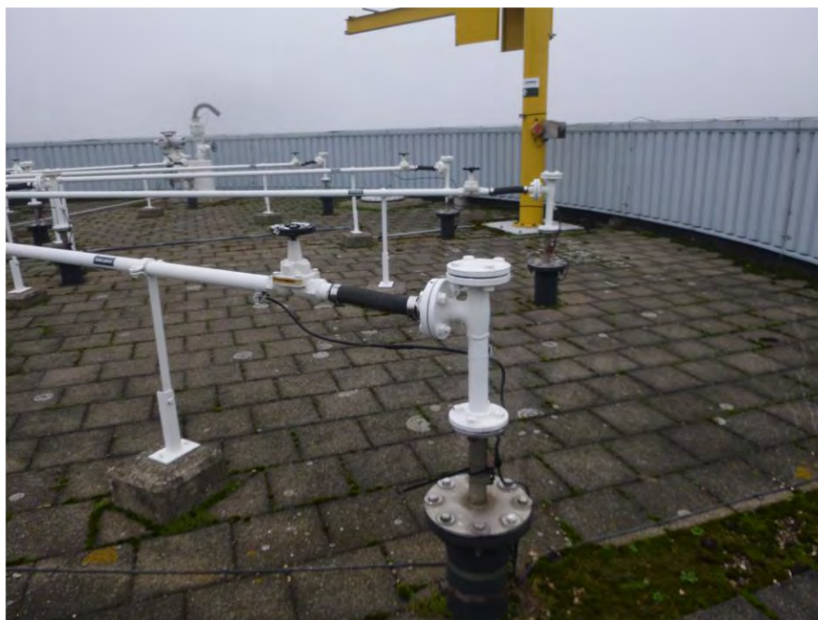
Foto F75, Coating - Slippistingstank 1 & 2
