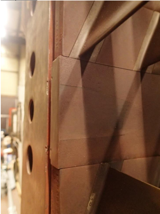
Quit heavy, old Rub Marks on Upper Half Compressor Casing R11
