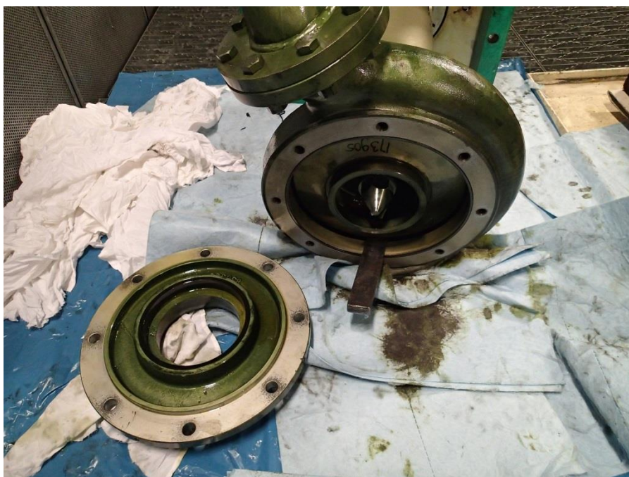
Auxiliary Lube Oil Pump
