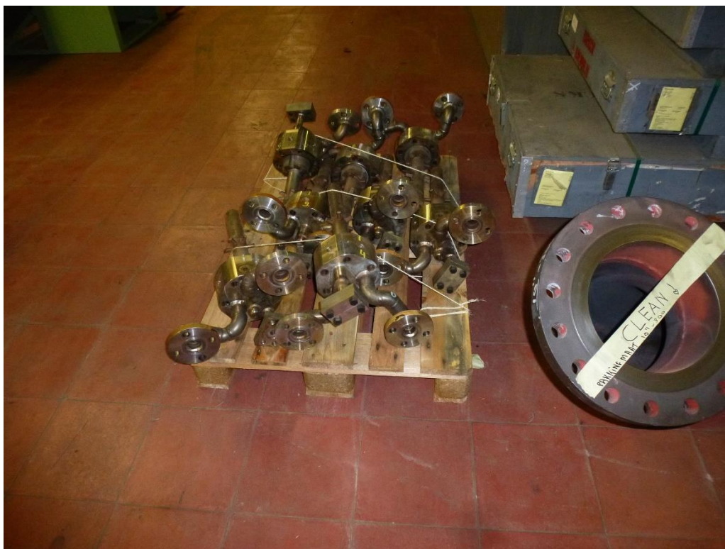
Disassembled Secondary burners
