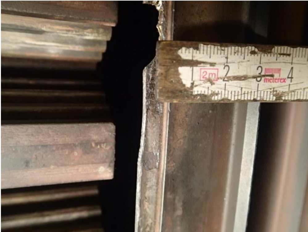
Damaged Discourager seal
