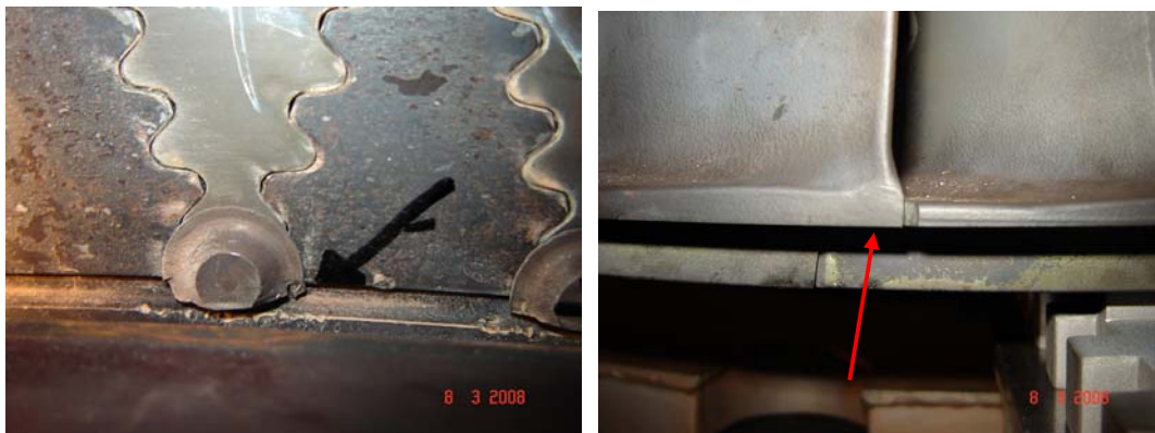
Detail of formerly damaged twistlock and no severe deflection noticed at tips
