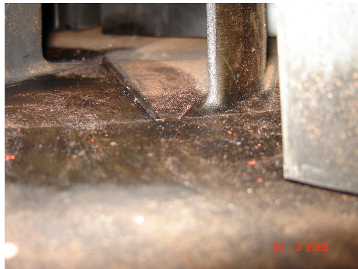
This shim was protruding into the flow path.
