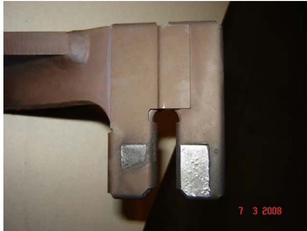
Wear of the hard metal contact surface
