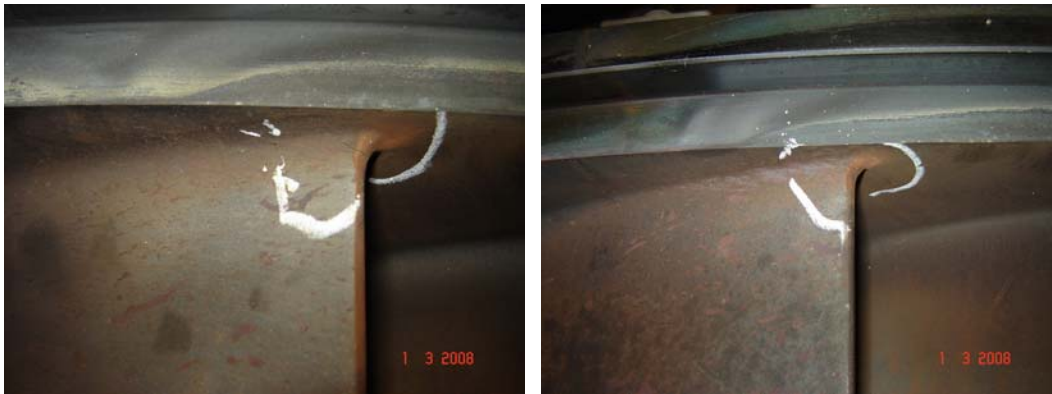
Light cracks at the corner of the vanes
