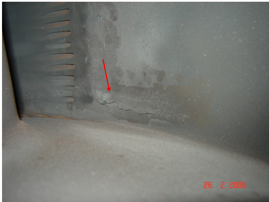
Some of the cracks in the vanes
