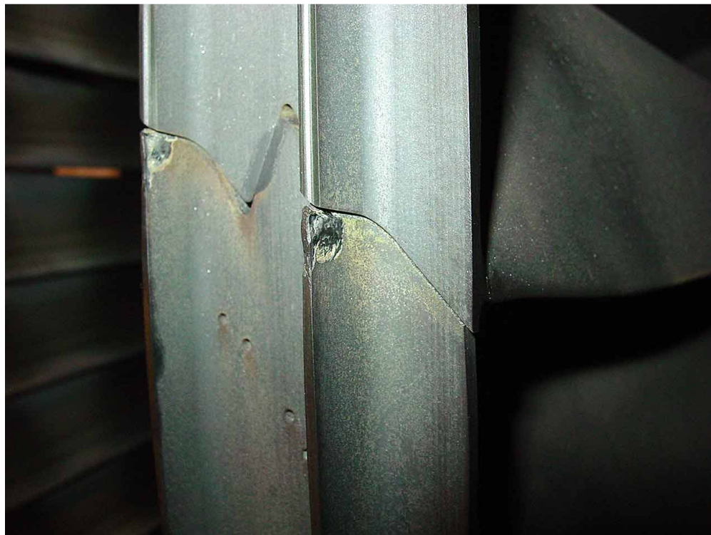
STG2 BUCKET SHROUDED TIP AND CUTTER TEETH DEFECTS
