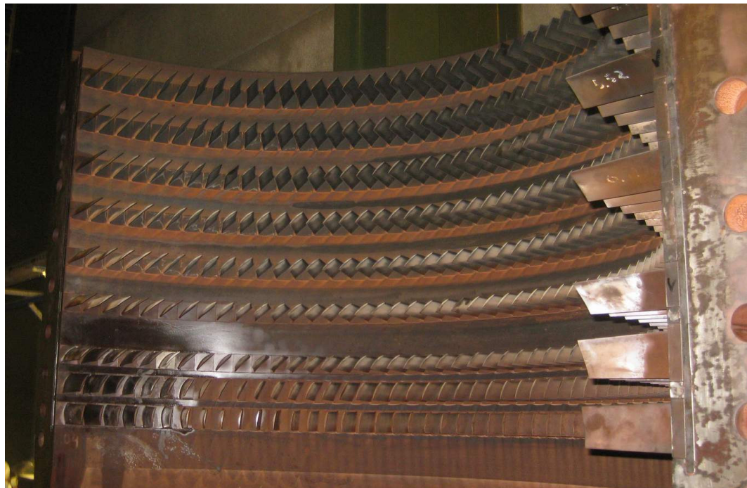
CDC COMPRESSOR STATOR VANE GENERAL GOOD CONDITION
