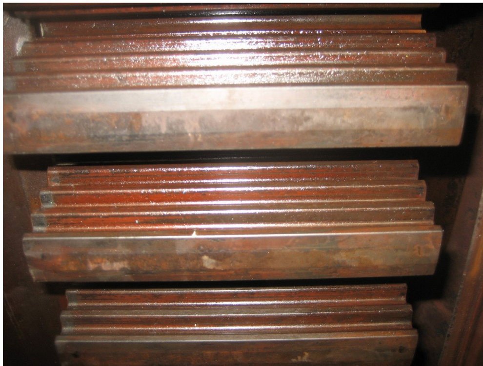
STG2 BUCKET DOVETAIL SLIGHTLY CORRODED
