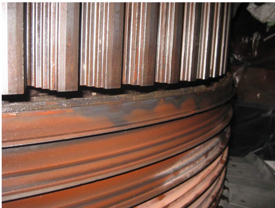
EVIDENCE OF HOT SPOT DISCOLORATION ON THE SPACER DUE TO FAULTY DISCOURAGER SEAL WHICH LEAKS HOT GAS
