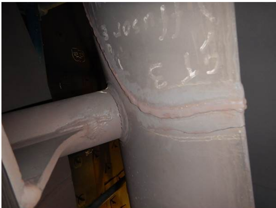
Scheurvorming in de diffusor
