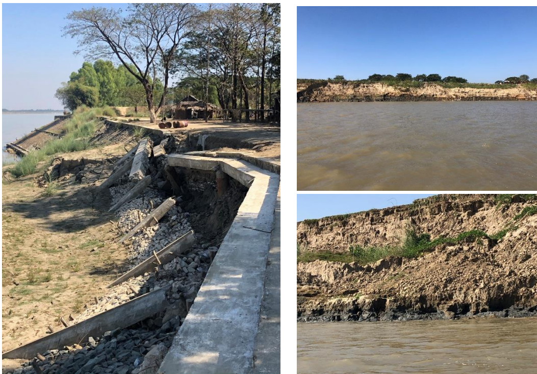
Figure 3 photos taken during field trip on 27 January showing serious erosion on west bank
